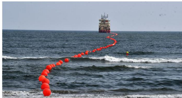
Powering up: More cables land in Singapore, a small city-state, than they do in all of India. FILE PHOTO
